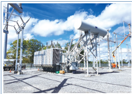
▲ 500kV 350MVA(Transformer(First Energy/USA))
