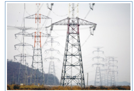
▲ Transmission Line Fittings(KEPCO/Dangjin)
