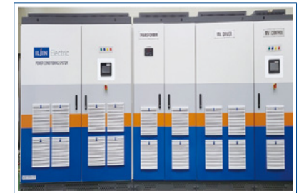
▲ Naju 5kV DC converter (500kW) in Jeollanam-do
