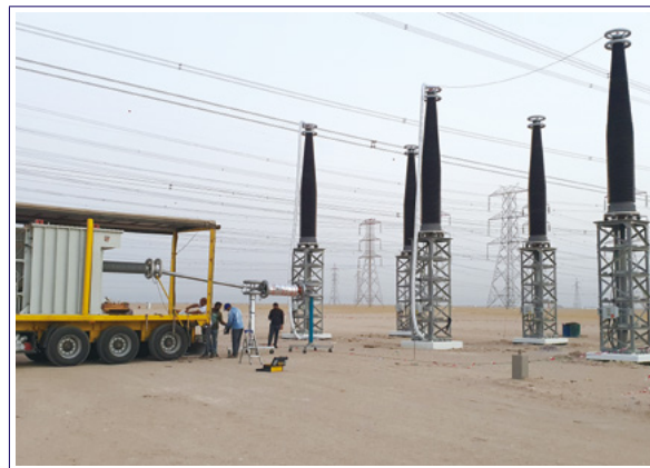
▲ 400kV Power Cables at Al-Mutla in Kuwait
