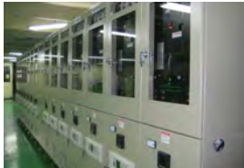
25.8/36kV GIS indoor Substation
