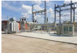
72.5kV GIS Outdoor substation
