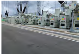
170kV GIS Outdoor substation
