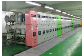
25.8kV E-GIS indoor substation
