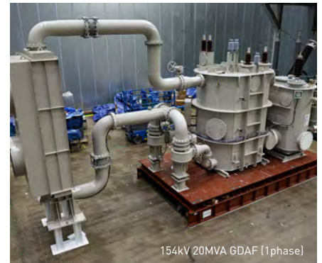
154kV 20MVA GDWF [1phase]
