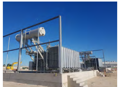
Australia, 3 PHASE 132kV 45MVA
