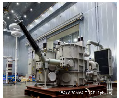
154kV 20MVA GDAF [1phase]
