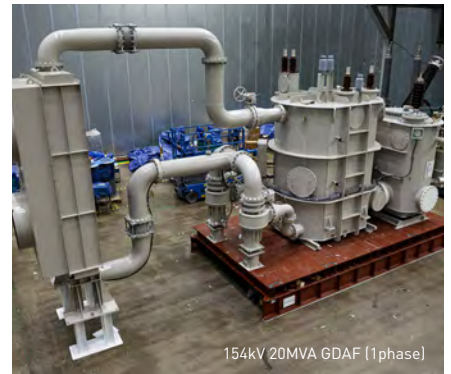
154kV 20MVA GDWF [1phase]
