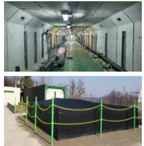
[ PQ test loop of 154kV PP insulated system ]
