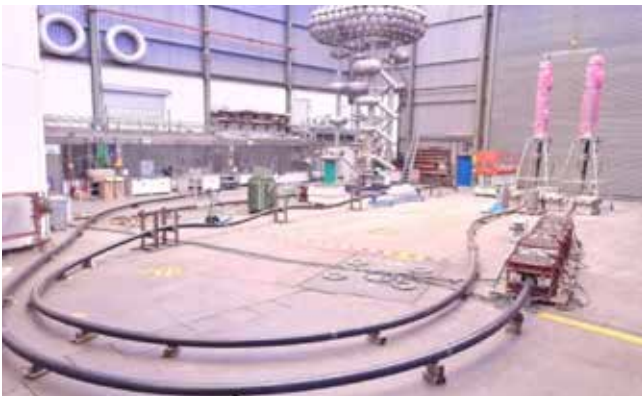
[ ±320kV VSC type XLPE cable system PQ test loop at KEMA FGH ]
